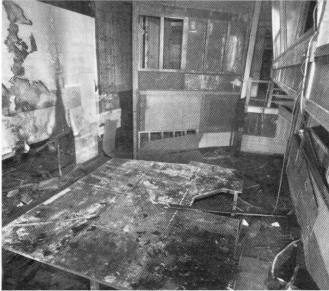
View of the plotting room after it had been closed and the vandals visited. The seat of the fire can be seen at the bottom of the map boards on the left of the picture. The sadly distressed plotting table fills the centre of the room.
